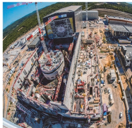
Construction of ITER (International Thermonuclear Experimental Reactor) in October 2018 (Cadarache in Saint-Paul-Lès-Durance, France) Source: ITER Organization
