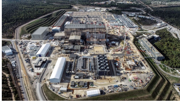
Construction of ITER (International Thermonuclear Experimental Reactor) in October 2021 (Cadarache in Saint-Paul-Lès-Durance, France) Source: ITER Organization
