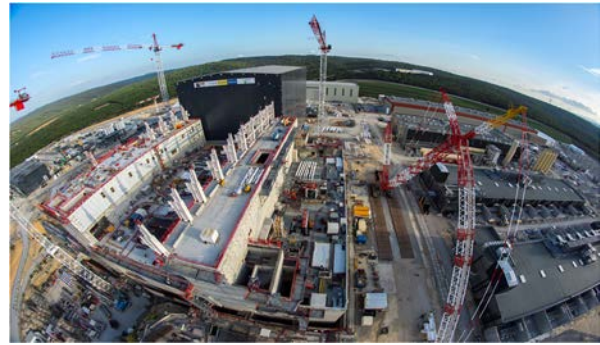
Construction of ITER (International Thermonuclear Experimental Reactor) in September 2019 (Cadarache in Saint-Paul-Lès-Durance, France) Source: ITER Organization
