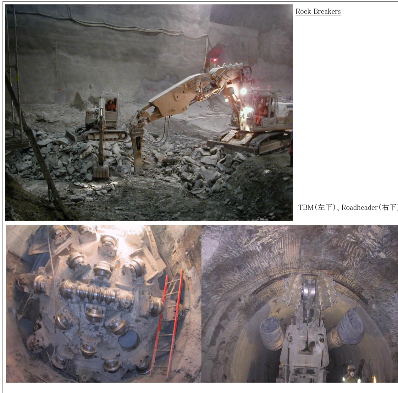
出典 ILC NRI CERN Visit 30 November 2017 Civil engineering aspects and challenges/John Osborne
