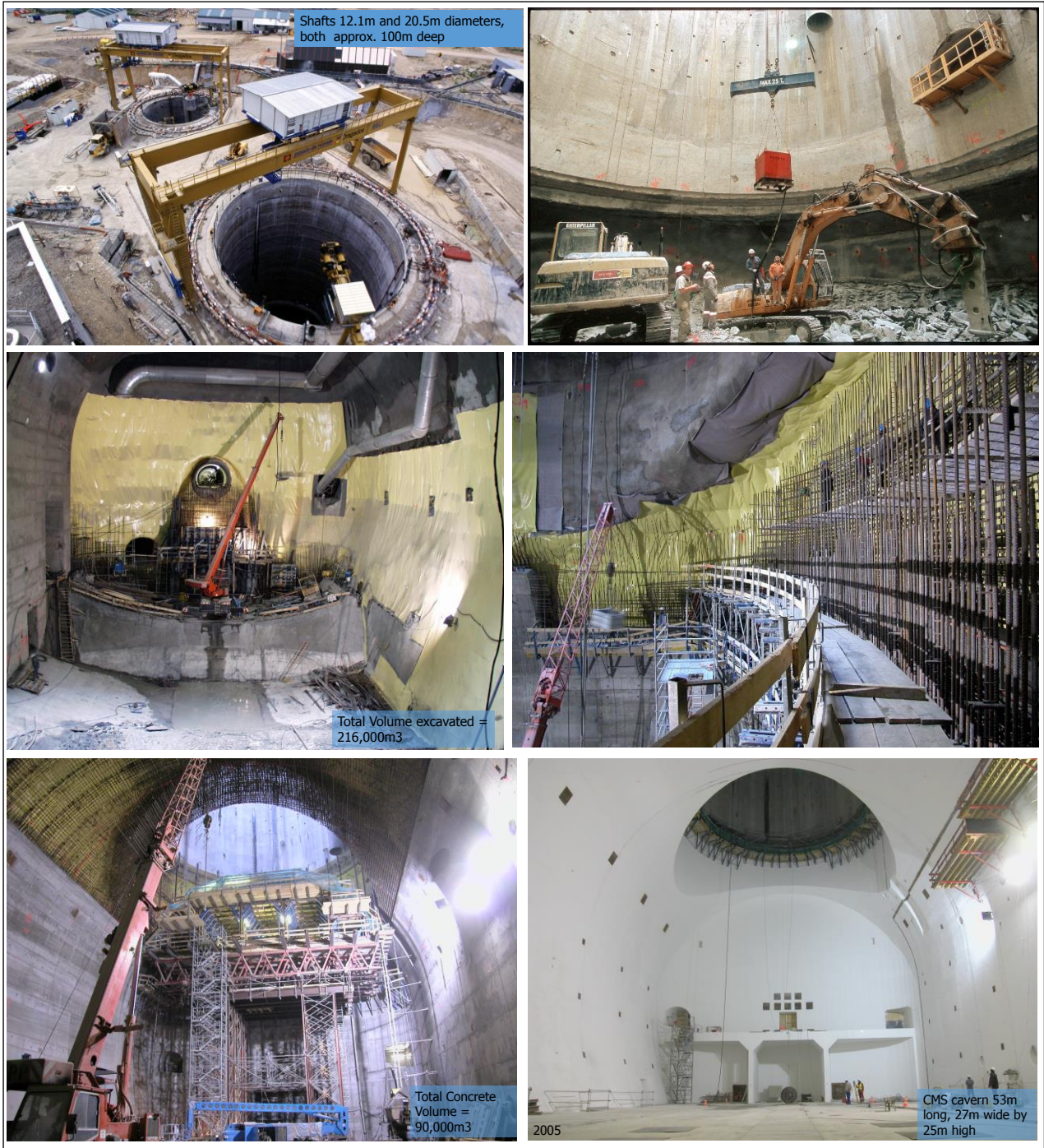
出典 ILC NRI CERN Visit 30 November 2017 Civil engineering aspects and challenges/John Osborne
